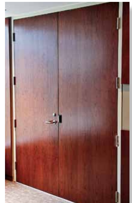
Acoustic Wood Doors & Steel Frame Conference Center
