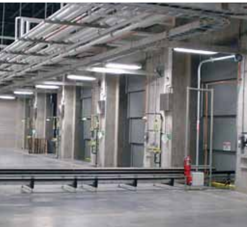
Overhead Blast Resistant Doors Pharmaceutical Plant
